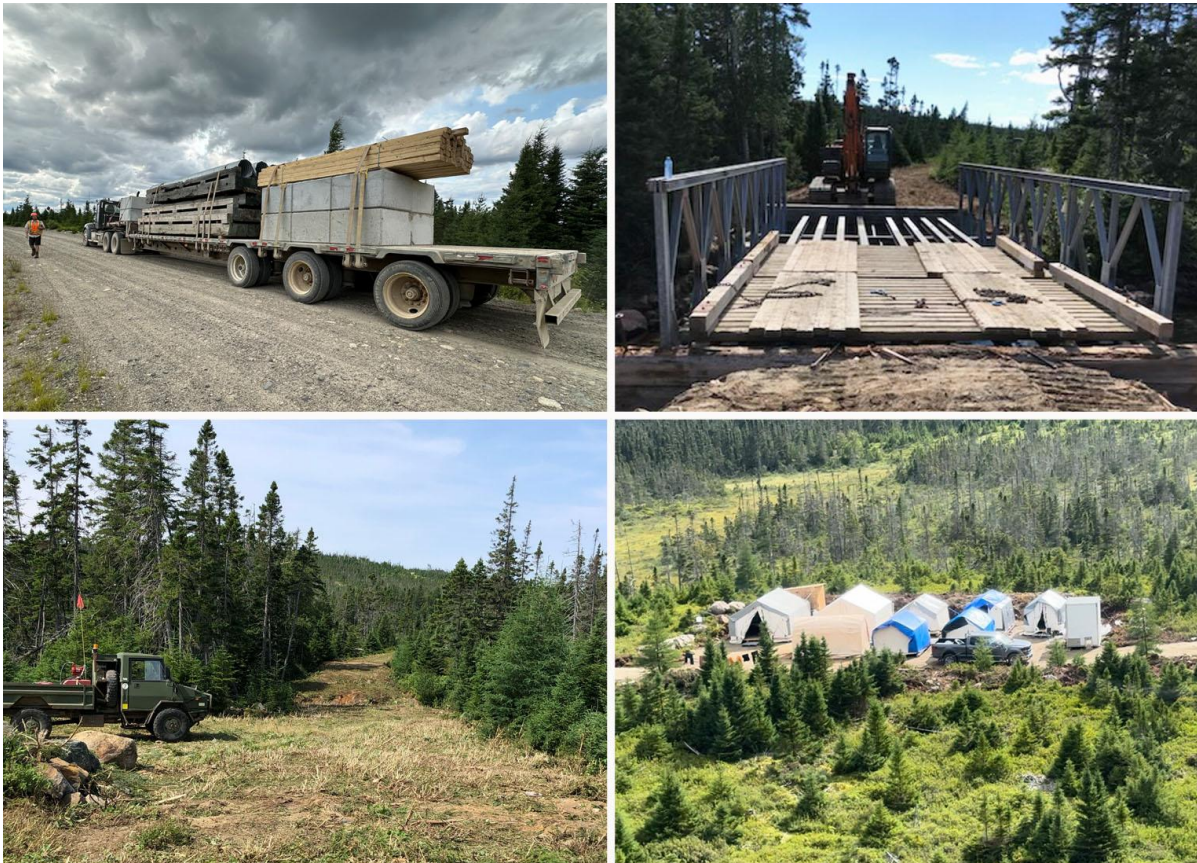
Figure 1: Images showing infrastructure upgrades including road clearing, culverts, and multiple bridge installations giving year round access to the Project. Bottom right, phase 1 camp established on the Atlantic Nickel Project site.
