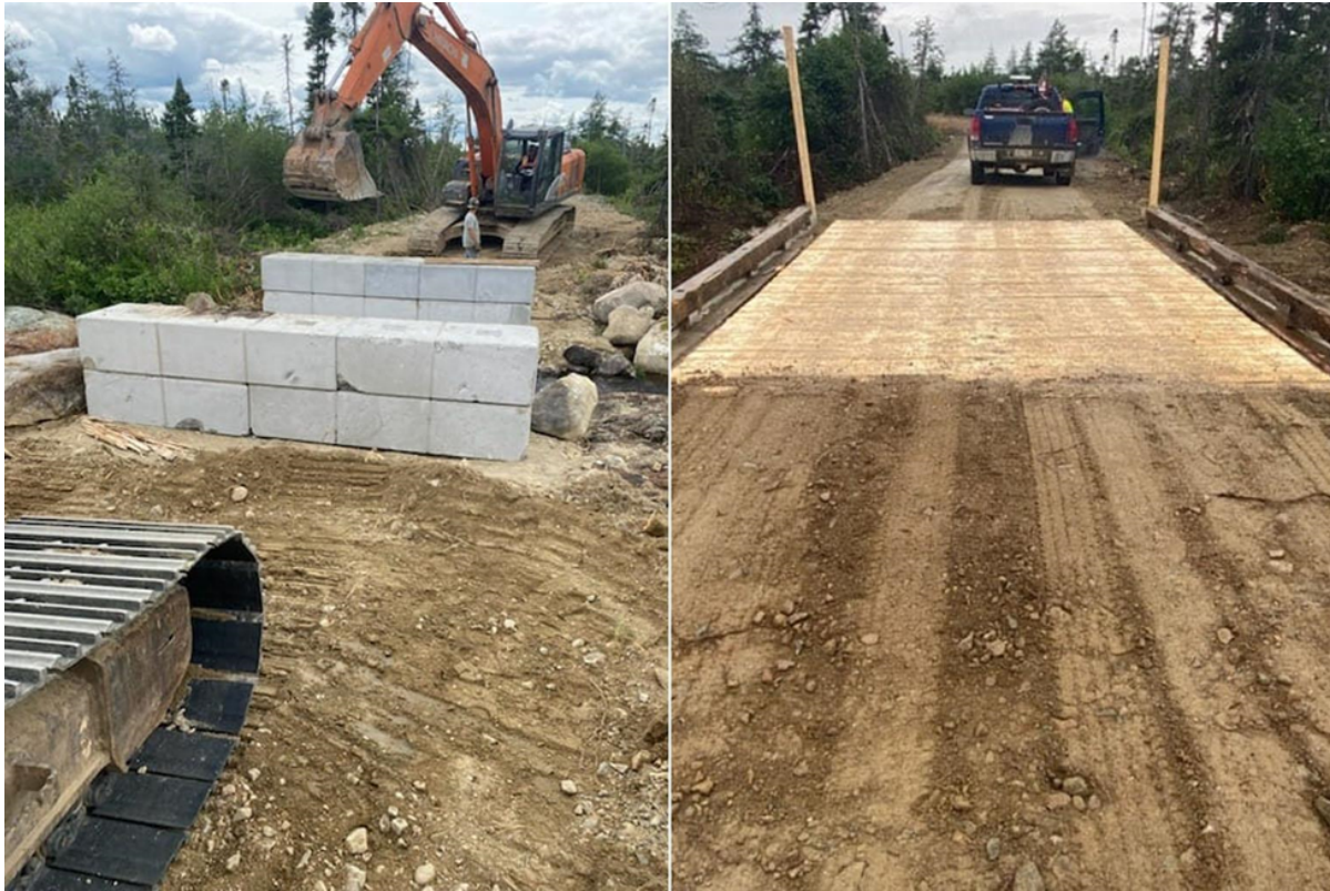
Figure 1: Bridge 1 completed at Atlantic Nickel Project, before (left) and after (right) as part of infrastructure upgrades.
